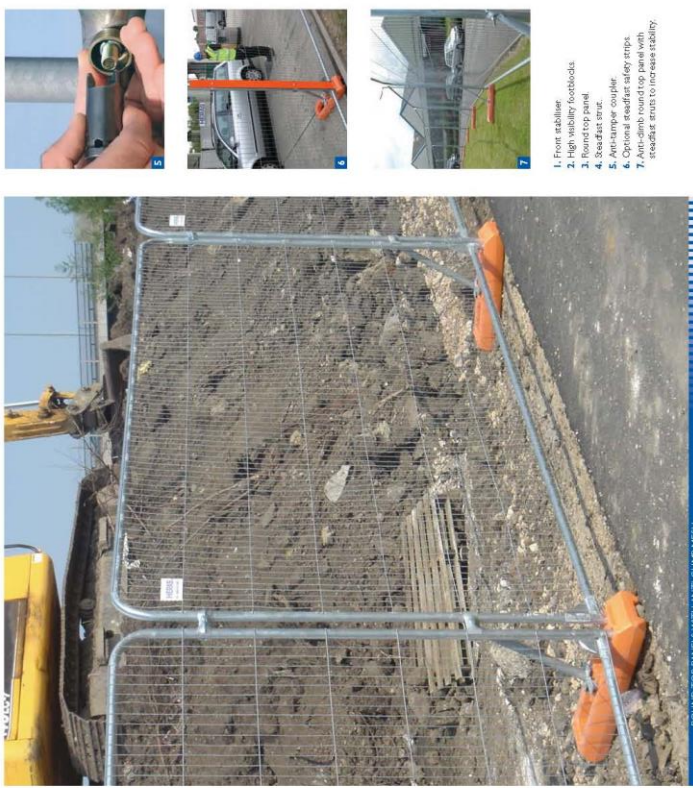
ROUND TOP PANELS WITH ANTI-TAMPER RESTR
